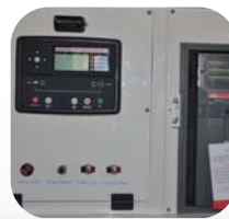
Control Panel & MCB
